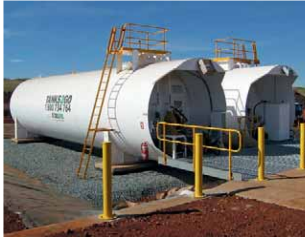
Tanks need to be self bunded.
