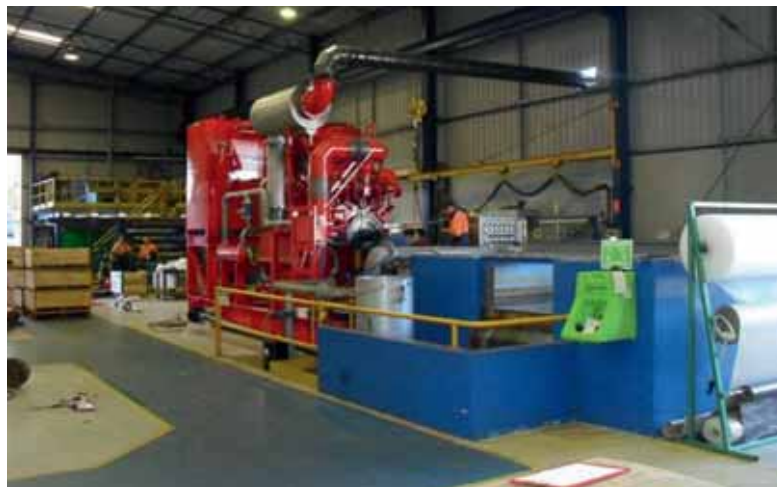
The test facility with a 1500 hp Zone2 specified fire deluge pump sent for testing.
